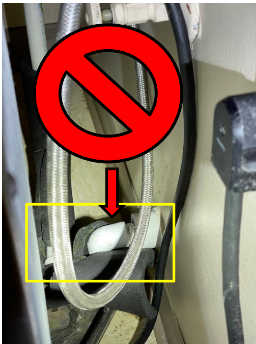
Ice Machine installed with No Airgap, Directly connected to Sanitary Sewer System.
