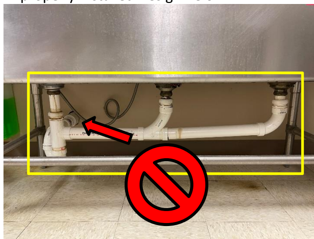
Three-Compartment Sink with No Airgap, Directly connected to Sanitary Sewer System.
