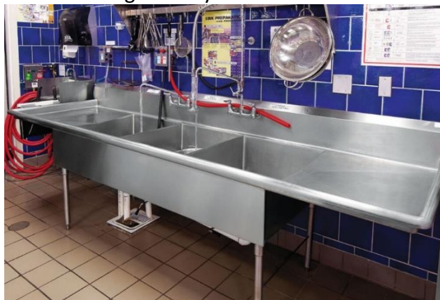
Three-Compartment Sink w/ Sanitary Sink
